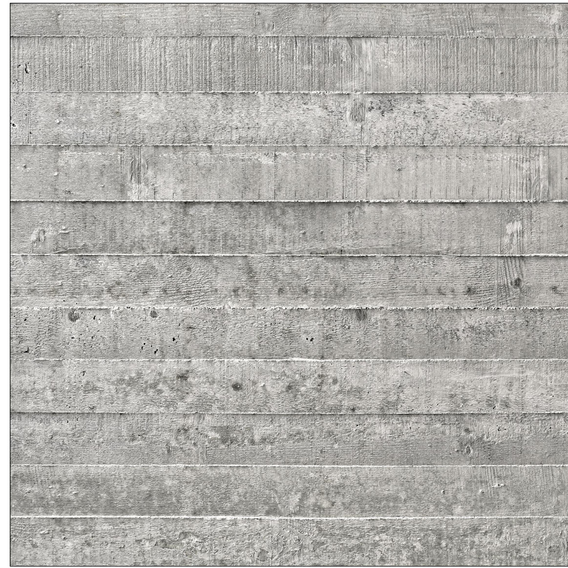
C BOARD-FORMED CONCRETE BUILDING ACCENT MATERIAL, SITE WALLS MANUFACTURER: BY GENERAL CONTRACTOR. MOCK-UP REQ'D
